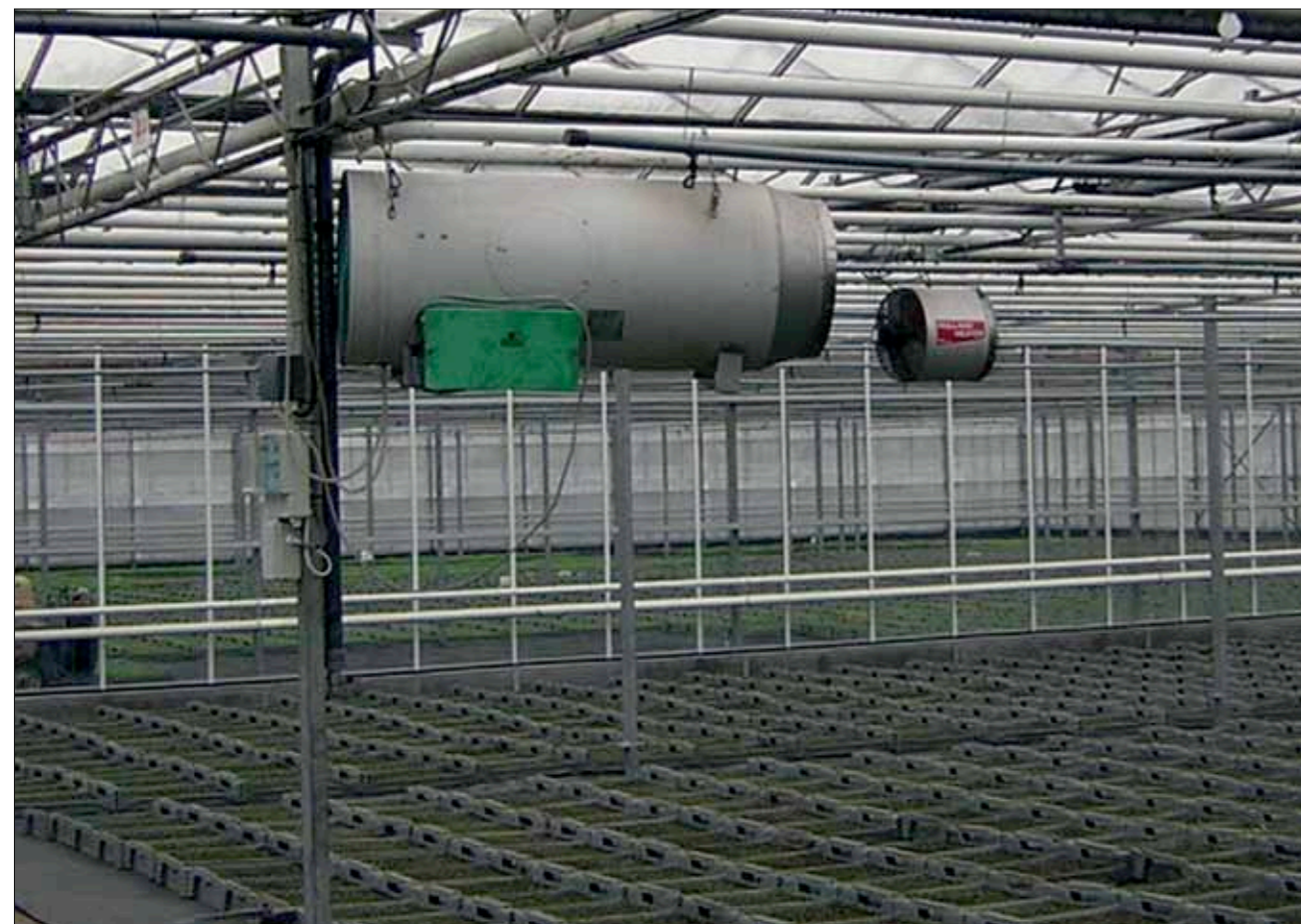
4 Air heater in use in a propagation house
