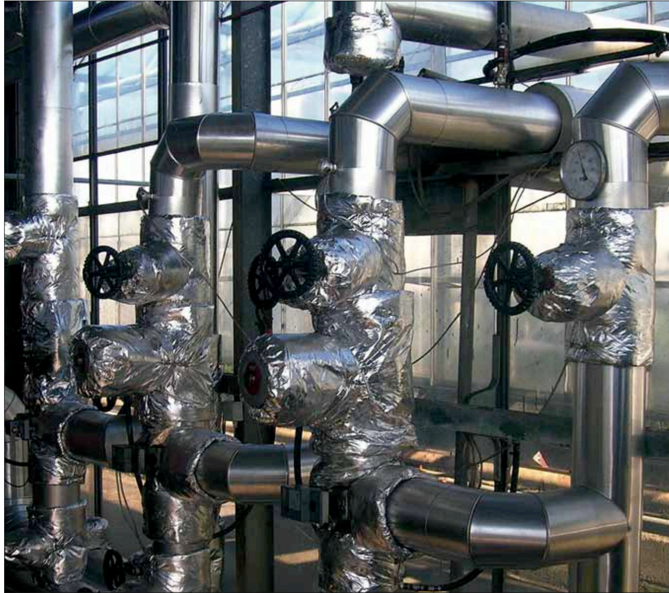
6 A good example of how flexible jackets can be used to insulate pumps and valves
